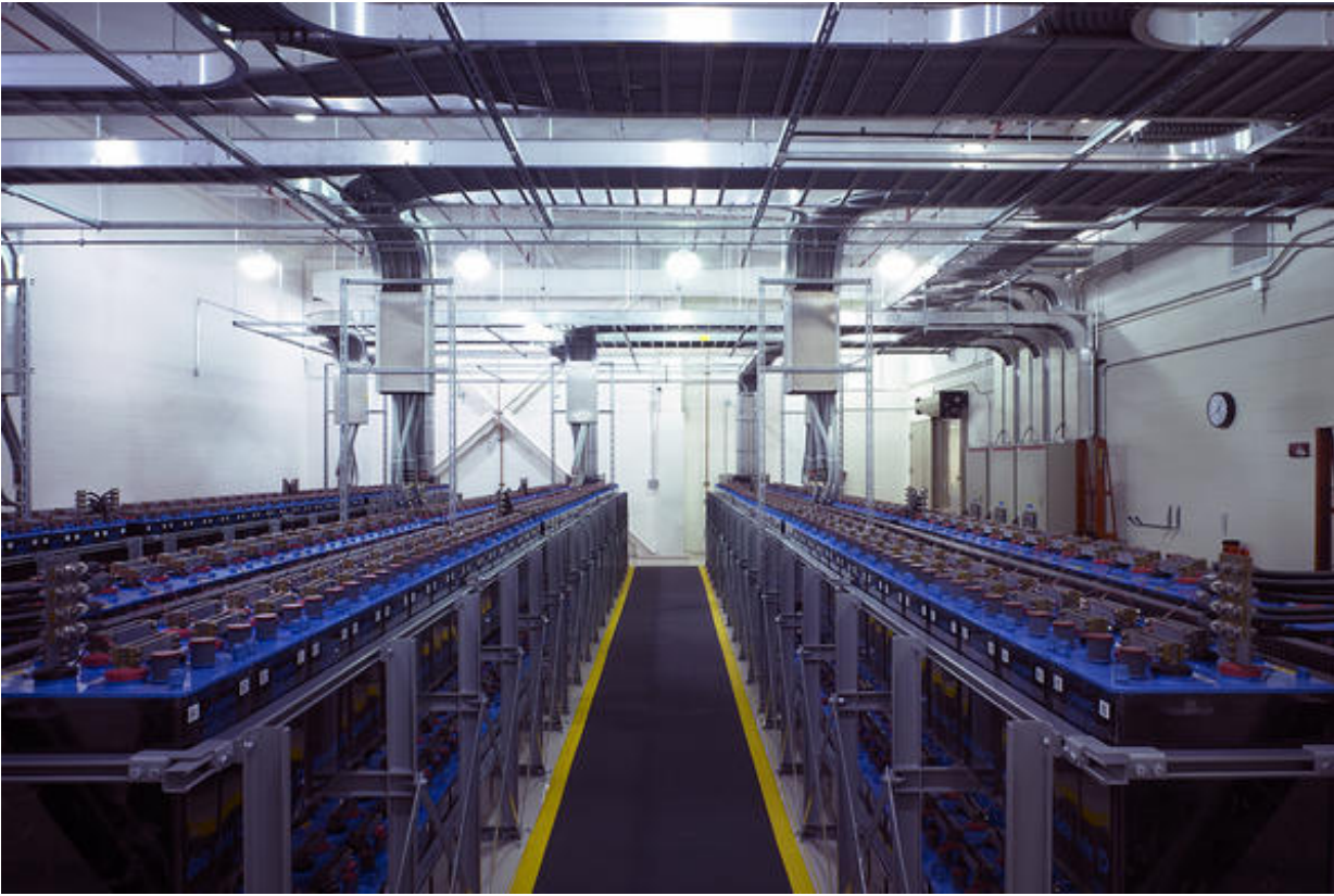
Blue Cross Blue Shield Data Center
