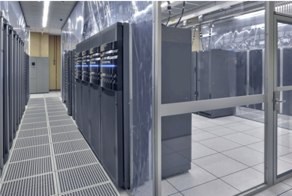
OSF Healthcare System Data Center
